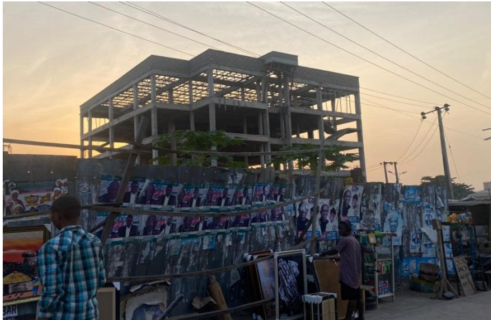
Plate 5: Abandoned Building Construction Project in Abeokuta. Source: Authors' Field Survey, 2024
